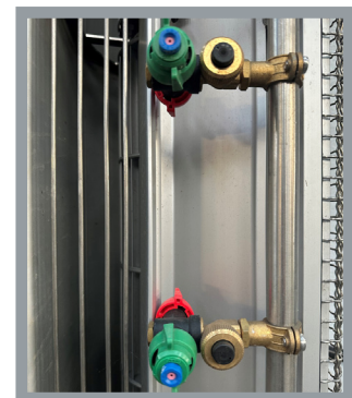
Fan with wet boom
